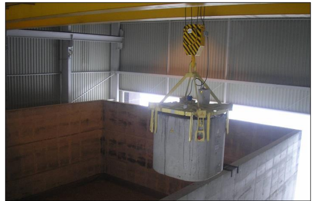
Radioactive waste package loading into ENSDF section
