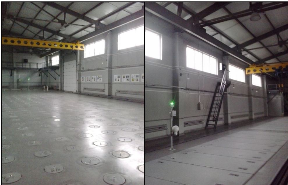
Area for storage of disused radiation sources at CLTSF
