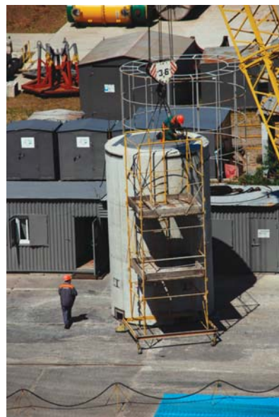
Ventilated concrete container (VCC) production site at the Zaporizhzhya NPP
