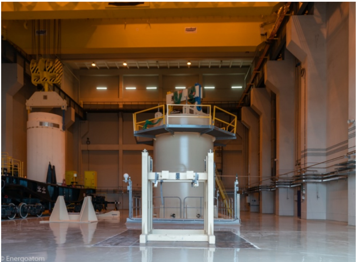
Photo 3. Central hall of the CSFSF container acceptance building
