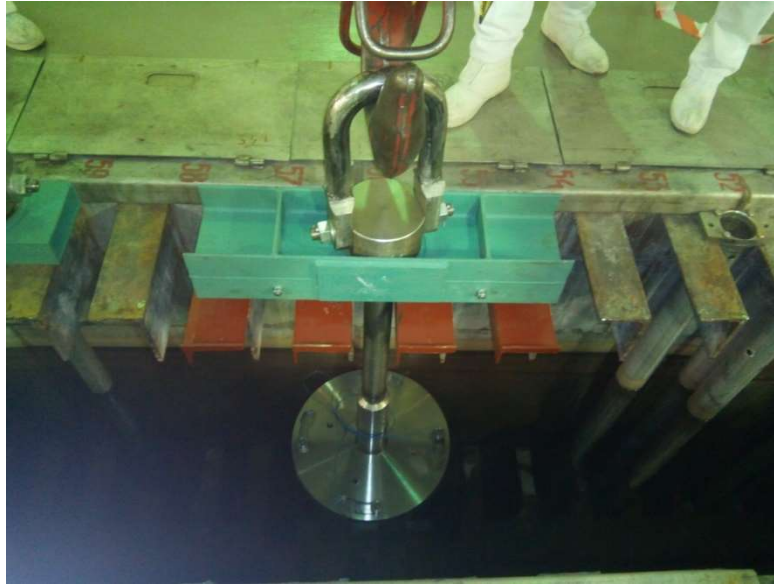
Figure 8.2 – Storage of damaged spent fuel in a unified canister/basket for special canisters in the ISF-1 canyon
